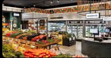
Commercial supermarket lighting
